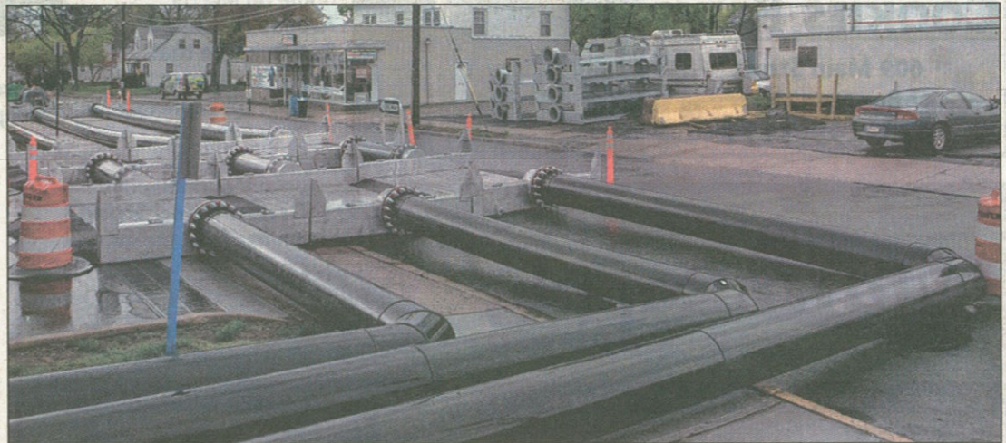
A labyrinth of sewer pipes line Monroe Street in Boonton as the Rockaway Valley Regional Sewerage Authority installation project is under way. It is expected to be completed by June.
