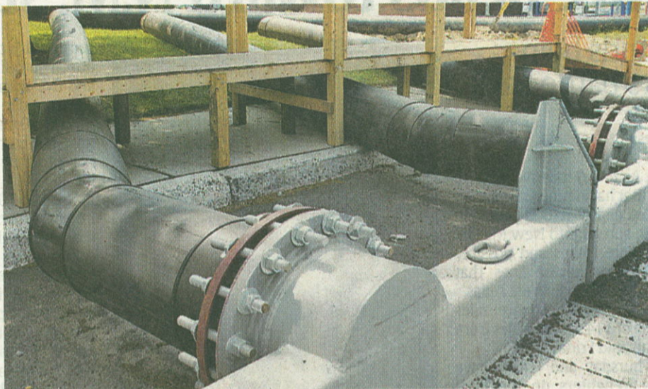
Temporary pipes, near the intersection of Washington and Monroe streets, handle sewage in Boonton this week. JUSTINA WONG/STAFF PHOTOGRAPHER
