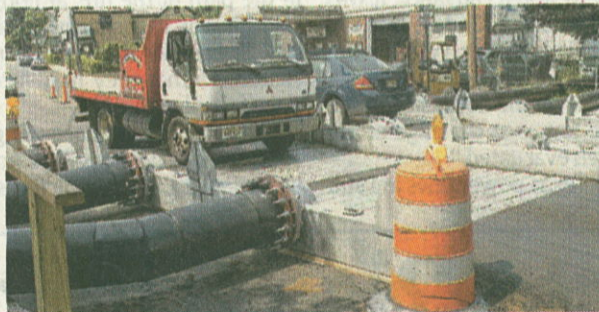
Traffic keeps flowing in downtown Boonton as work on a sewage pipe relining project continues. Temporary pipes have been removed on a portion of Monroe Street.
